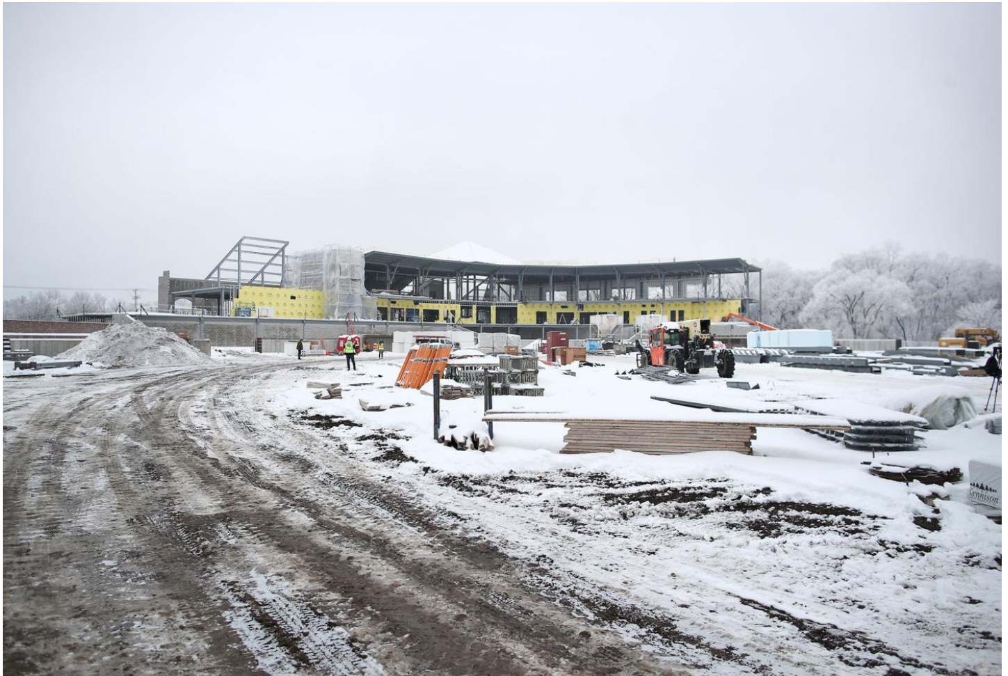
Construction on ABC Supply Stadium, located in downtown Beloit, continues and remains on schedule for a mid-summer opening in 2021.
